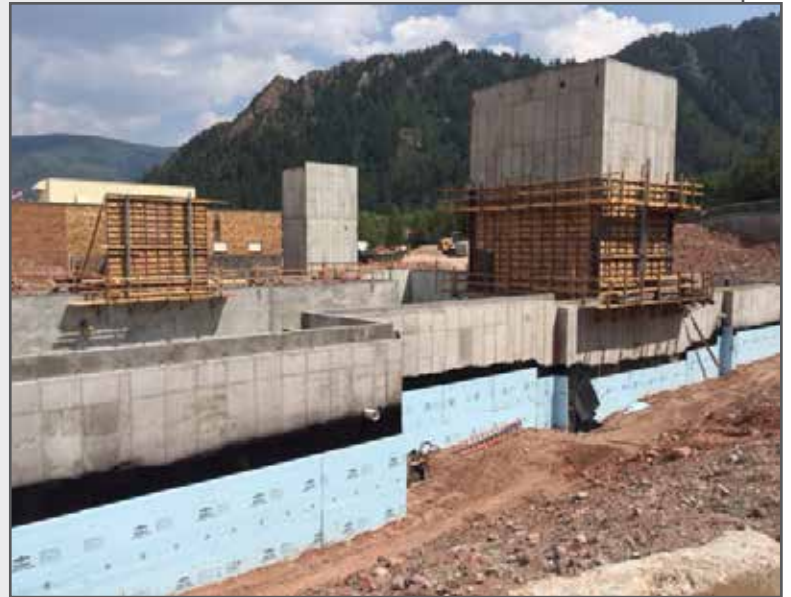
After months of earthmoving and site work, footers and foundations have been poured. The tall structures represent two elevators — one from the ER to the rooftop helipad and one from the new lobby to the second floor.
